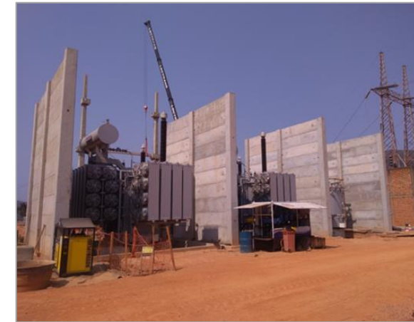
Barreiro Substation (1) Investment of R$ 115 million
