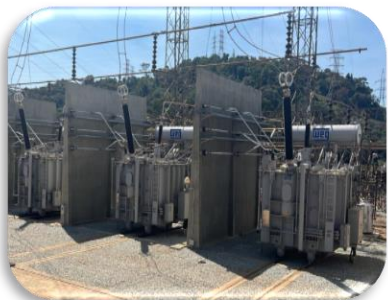
SE Taquaril New transformers
