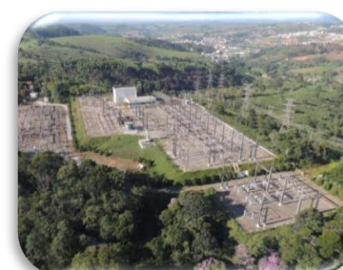
SE Lafaiete New equipment
