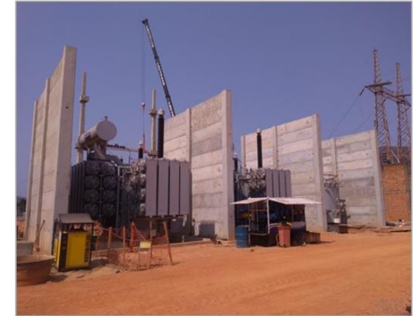
Barreiro Substation (1) Investment of R$ 115 million
