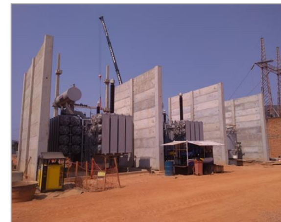
Barreiro Substation (1) Investment of R$ 115 million
