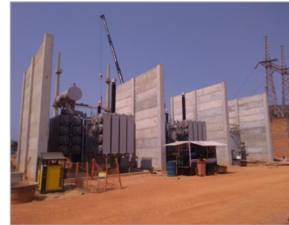
Barreiro Substation (1) Investment of R$ 115 million
