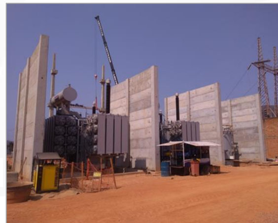
Barreiro Substation (1) Investment of R$ 115 million
