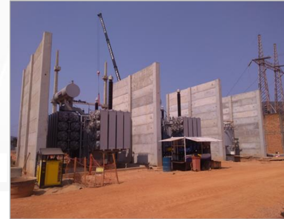
Barreiro Substation (1) Investment of R$ 115 million
