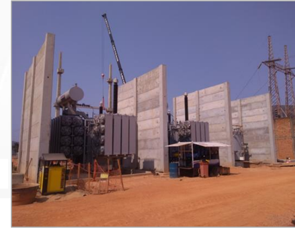
Barreiro Substation (1) Investment of R$ 115 million
