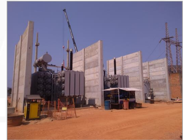
Barreiro Substation (1) Investment of R$ 115 million
