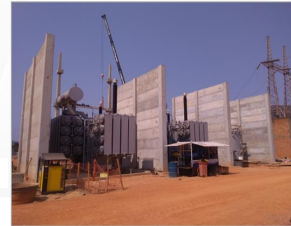
Barreiro Substation (1) Investment of R$ 115 million
