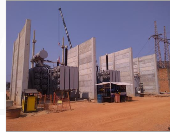
Barreiro Substation (1) Investment of R$ 115 million
